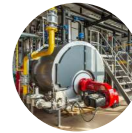
Chemicals for boilers
